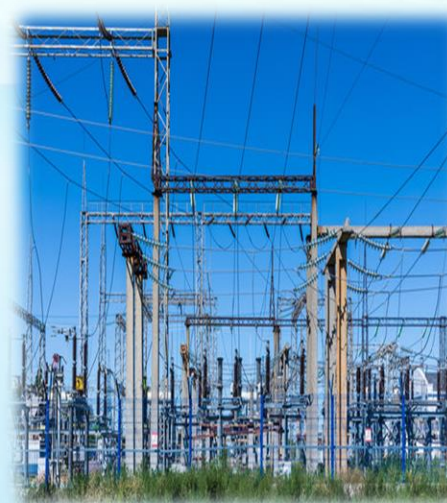
Number Of Station Transformers -Main 86 - Added sub(in2025): 237
