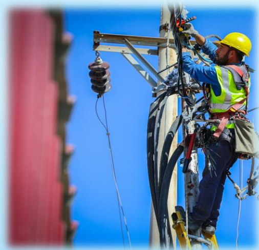
Added Low Voltage Network lengths 537.6 KM
